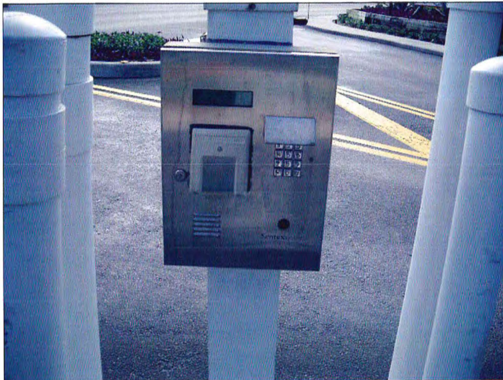
Access Control Entrance Keypad
