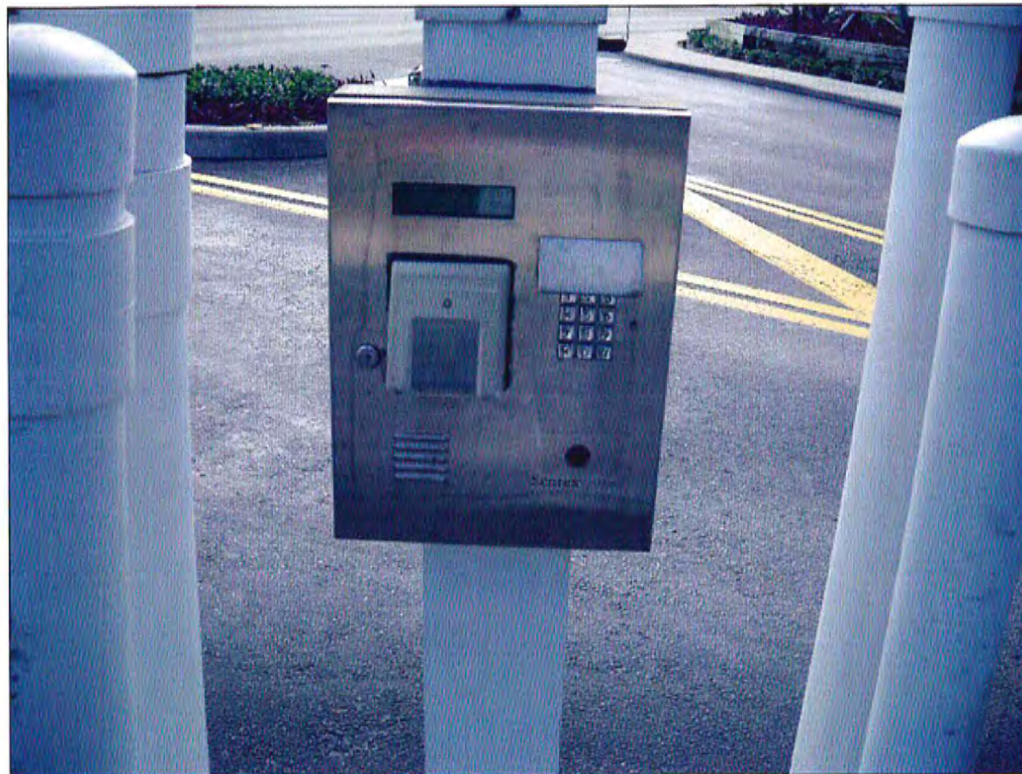
Access Control Entrance Keypad
